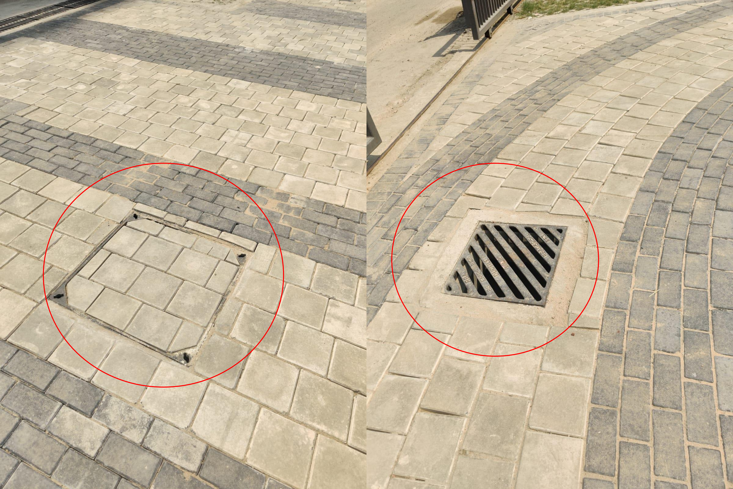
Internal Sewer & Storm water Line
